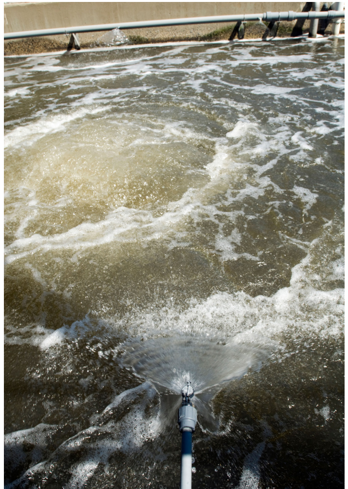
Sewage treatment - aeration
